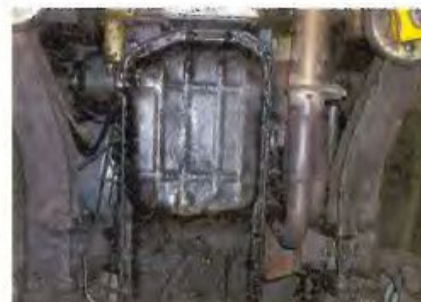
The whole chassis needs to be carefully inspected for any signs of corrosion...
